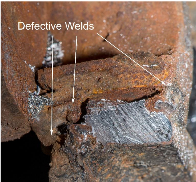
Figure 7 – Defective Welds Right Side - Rear Connection after Bracket Removal
