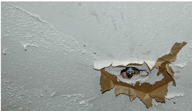
Figure 1 – Location of Failed Sprinkler
