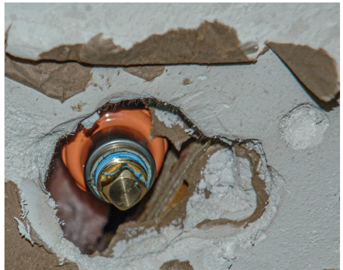
Figure 2 – Plug Replacing Failed Sprinkler
