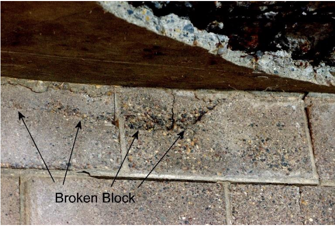
Figure 6 – Tipped and Broken Block
