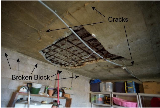
Figure 5 – Location of Garage Floor/Ceiling Collapse
