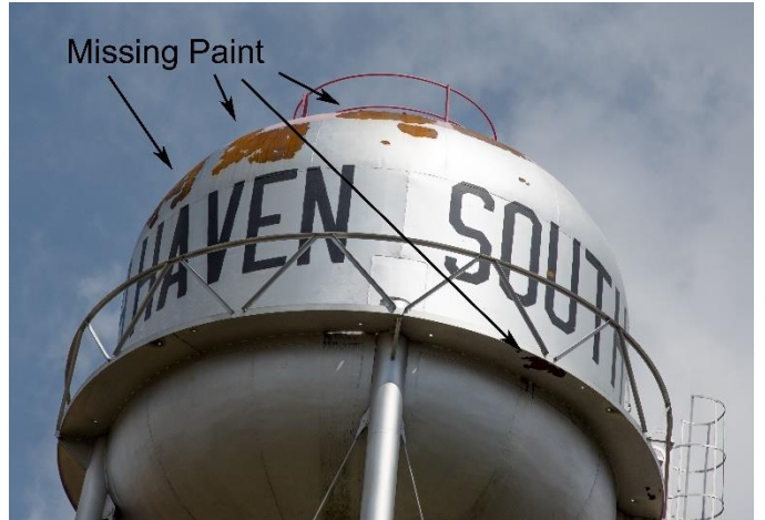
Figure 2 – Missing Paint on Top of Water Tower
