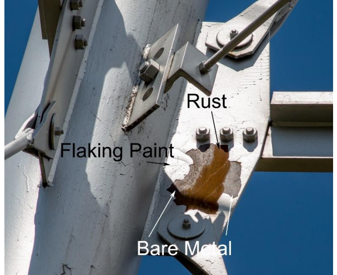
Figure 5 – Flaking Paint on Leg Tower Bracket
