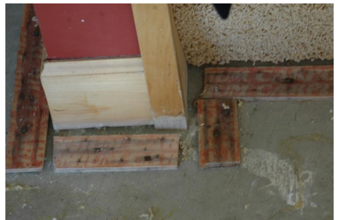
Figure 17 – Water Damage to Basement Woodwork
