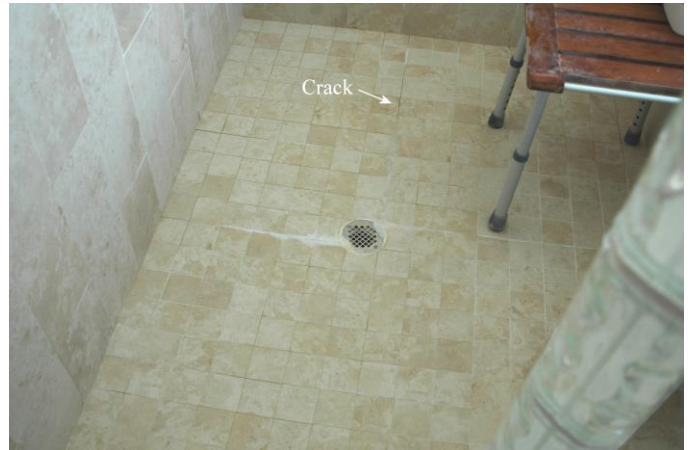
Figure 19 – Cracks in Grout, Master Bathroom Shower, Main Level
