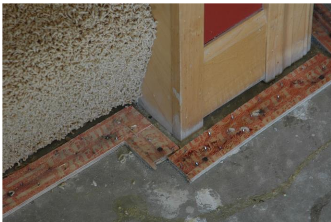
Figure 16 – Water Damage to Basement Woodwork
