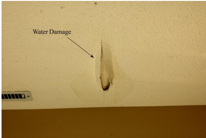
Figure 18 – Water Damage Ceiling, Southwest Basement Bedroom
