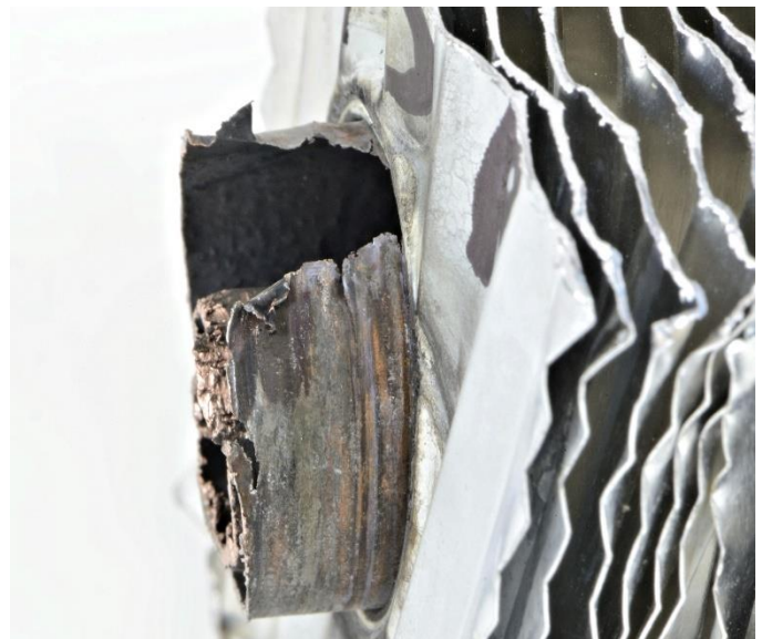
Figure 27 – Leak in Coil Sample 2
