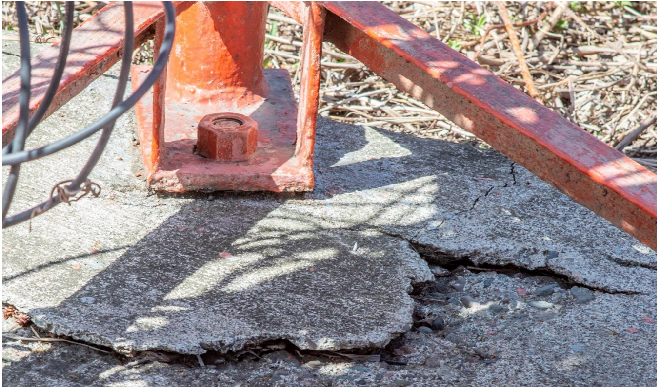
Figure 8 – Cracked Concrete Base North Leg
